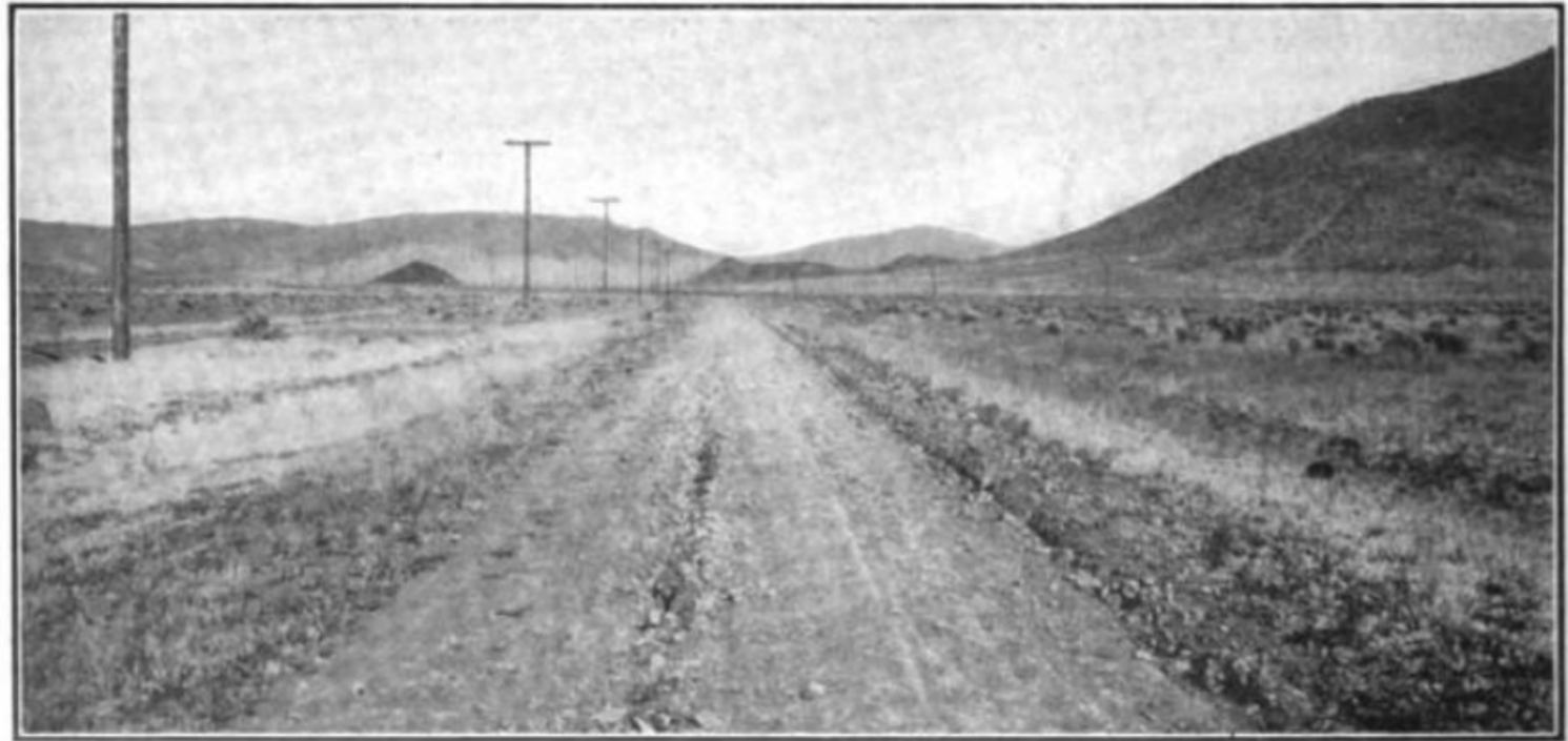
ROAD MONEY GOING TO WASTE AT MONTAGUE, CAL., WHERE AN EXPENSIVE MACADAM TRAP ROAD IS CRUMBLING INTO A MERE ROCK HEAP FOR LACK OF MAINTENANCE
